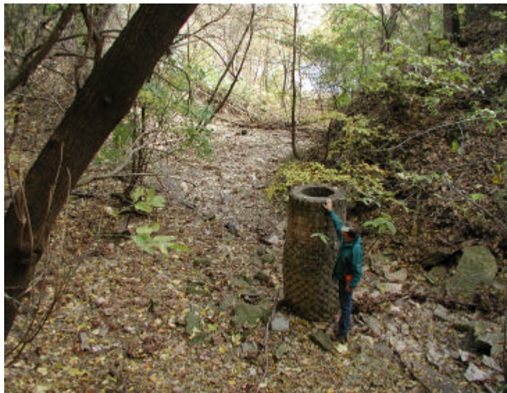
Figure 10. Erosion exposed this manhole in the ravine near 36 th Street.
